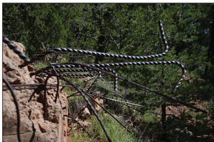
Photo of the culvert ruin above on the original alignment. Note the old style twisted steel rebar.
