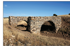
The remains of the NOTR culvert stand roughly 8 feet tall.
