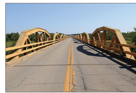
The William H. Murray "Pony" bridge, consisting of thirty-eight 100' long steel pony trusses stretching 3/4 of a mile in length. This bridge replaced the Key suspension bridge featured on Map 82. The Pony Bridge was reconstructed using the original trusses in 2022-2023.
