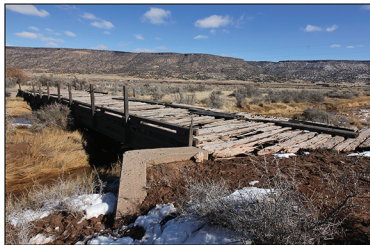
This timber bridge with concrete abutments (lower right of map) is nearly identical to the bridge on Map 89.
